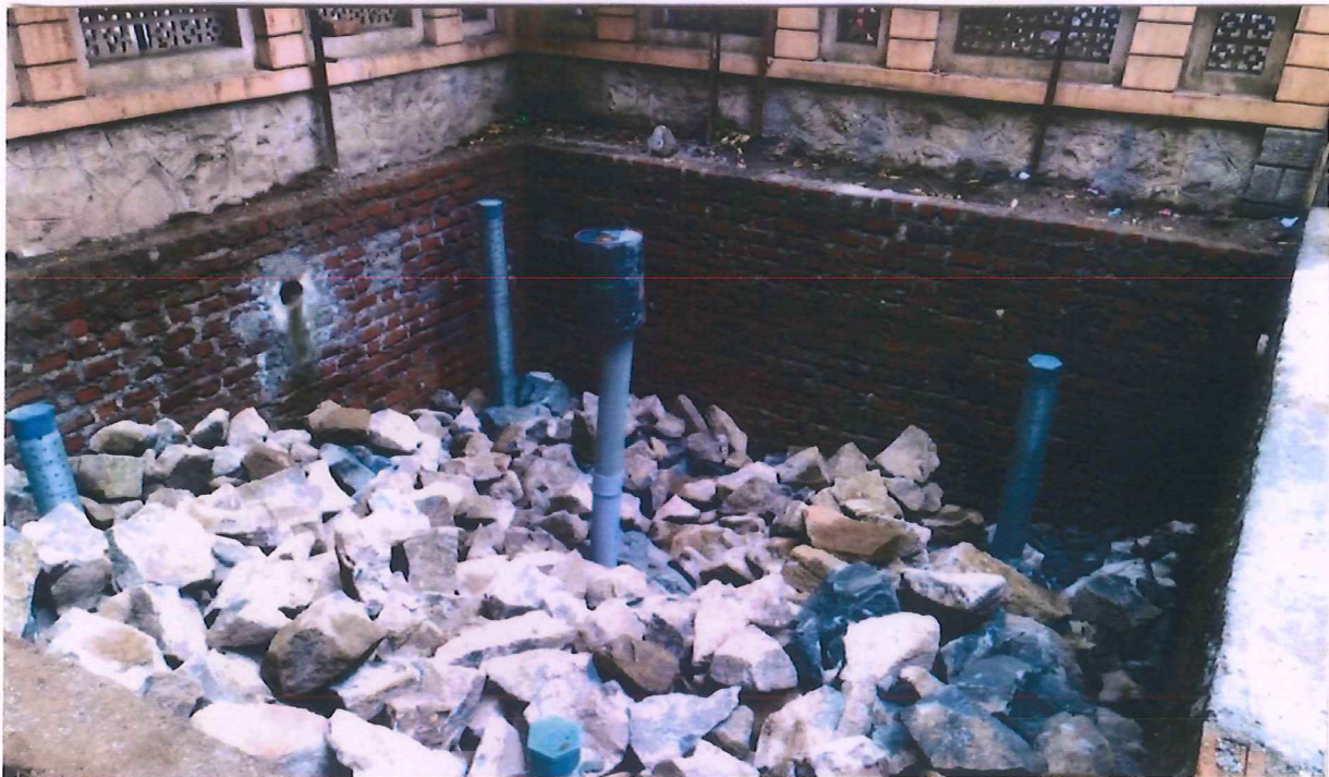
Rain water Harvesting plant SBES college of Art's & commerce, Aurangabad (MS)
